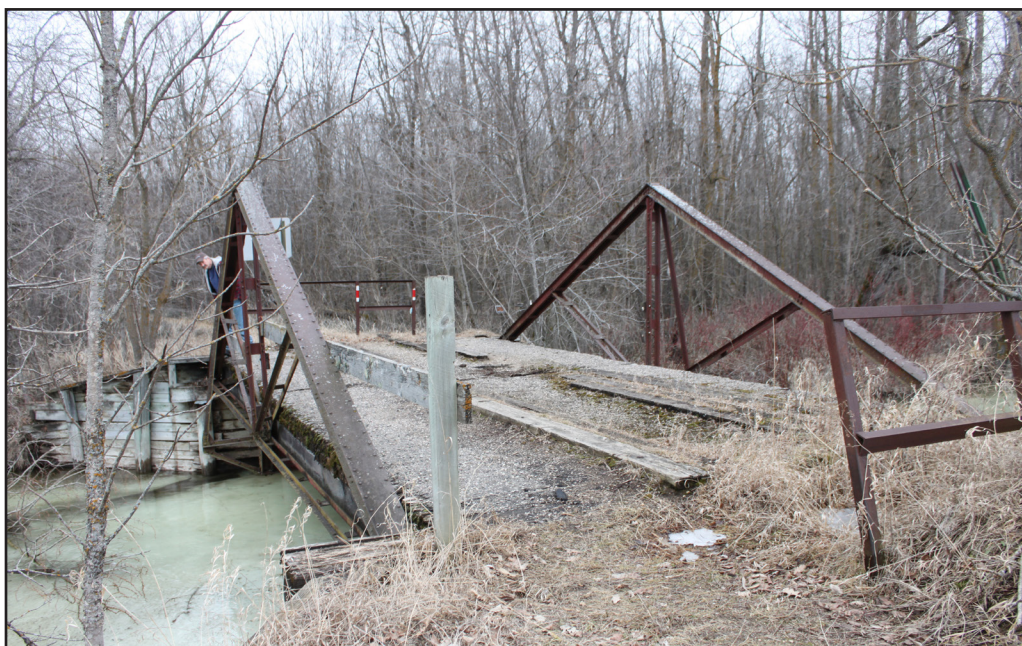
The Greenwood Bridge on its original site in Greenwood Township prior to being uprooted and moved to the LIRPF grounds last year. Now it is ready to support trains full of passengers on the North Itasca Railroad on the showgrounds.
